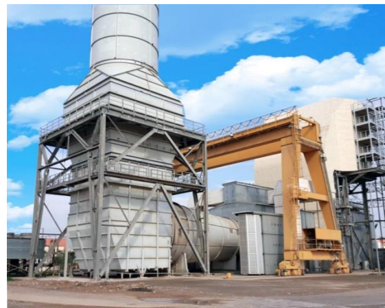
Figure 2. Kirkuk gas power station.[13]
