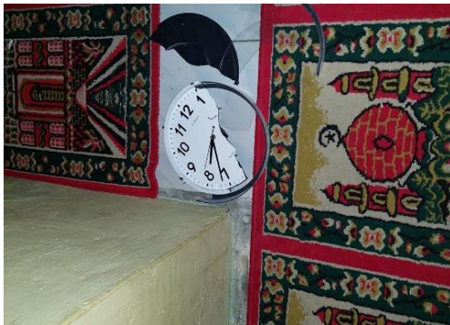
Fig.4. Visual Observation of clock fallen at earthquake time shaking
