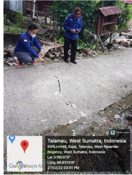
Fig.12. Ground failure at residential area Kajai Village
