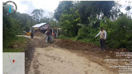
Fig.10. Broken Road at Talu Village
