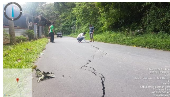
Fig.9. Ground Cracking at Talu Village
