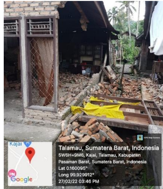
Fig.5. Damaged House at Kajari Village
