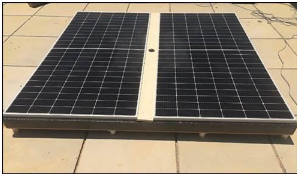
(b) PV solar installed on the base of the system
