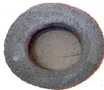
Figure 2: Air Diffuser of Inverse U shape
